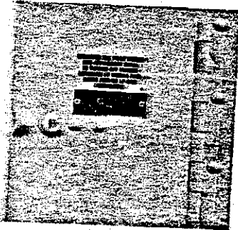
Figure 8-1. Generator Gas Tank Access Panel
