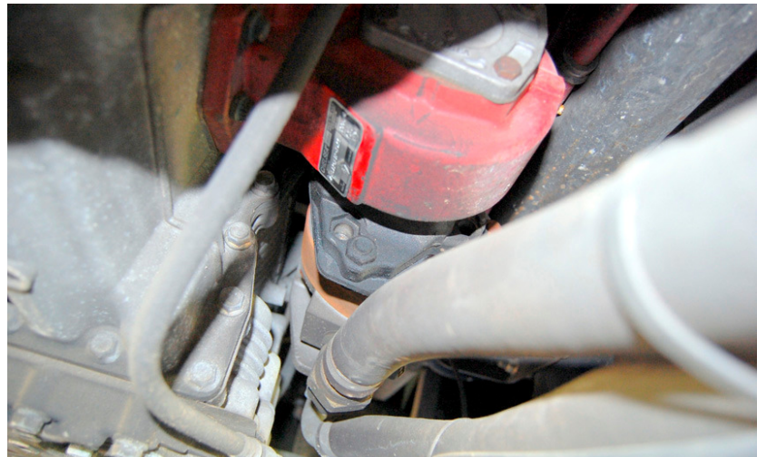
PTO with two pumps on passenger side of coach.
